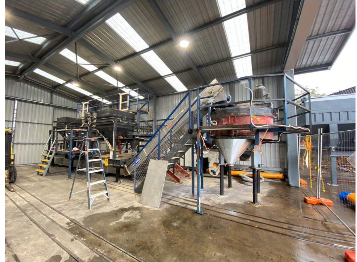
UniqueCem Mixing Plant at Vales Point (5,000 tpa, commissioned Sept 2024)
